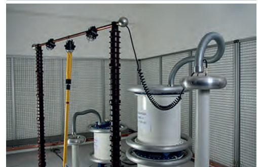
High voltage laboratory
